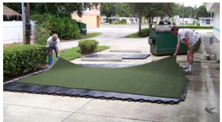
Turf is assembled onto the panels and stretched and stapled around the perimeter only. Turf can always be loose laid for temporary installations
